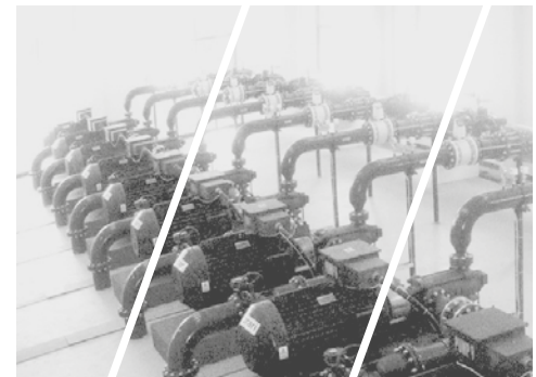
Boosting and Distribution of surface water
