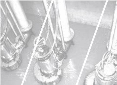
Wastewater Transport and Treatment
